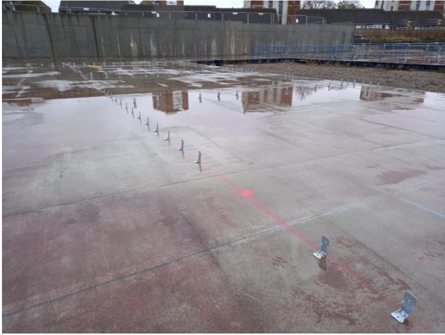
Brackets installed on lower ground floor slab ahead of cross laminated structure
